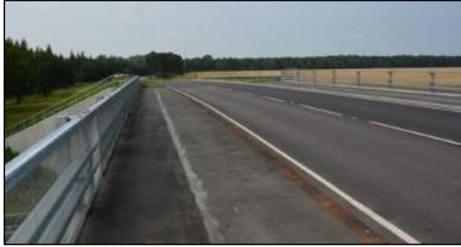
Figure E21. Looking across the top of the overbridge from the south east.
