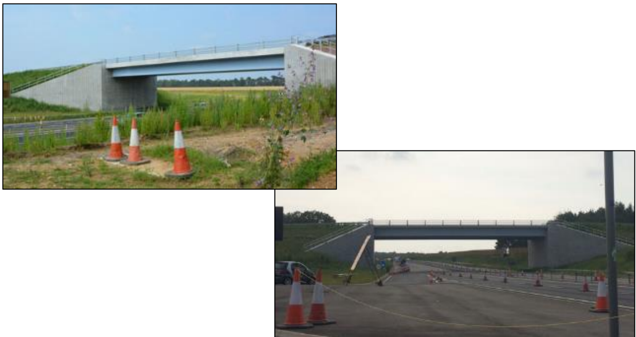
Figure E20. Side views of the overbridge taken from the south east (above) and north (below right).
